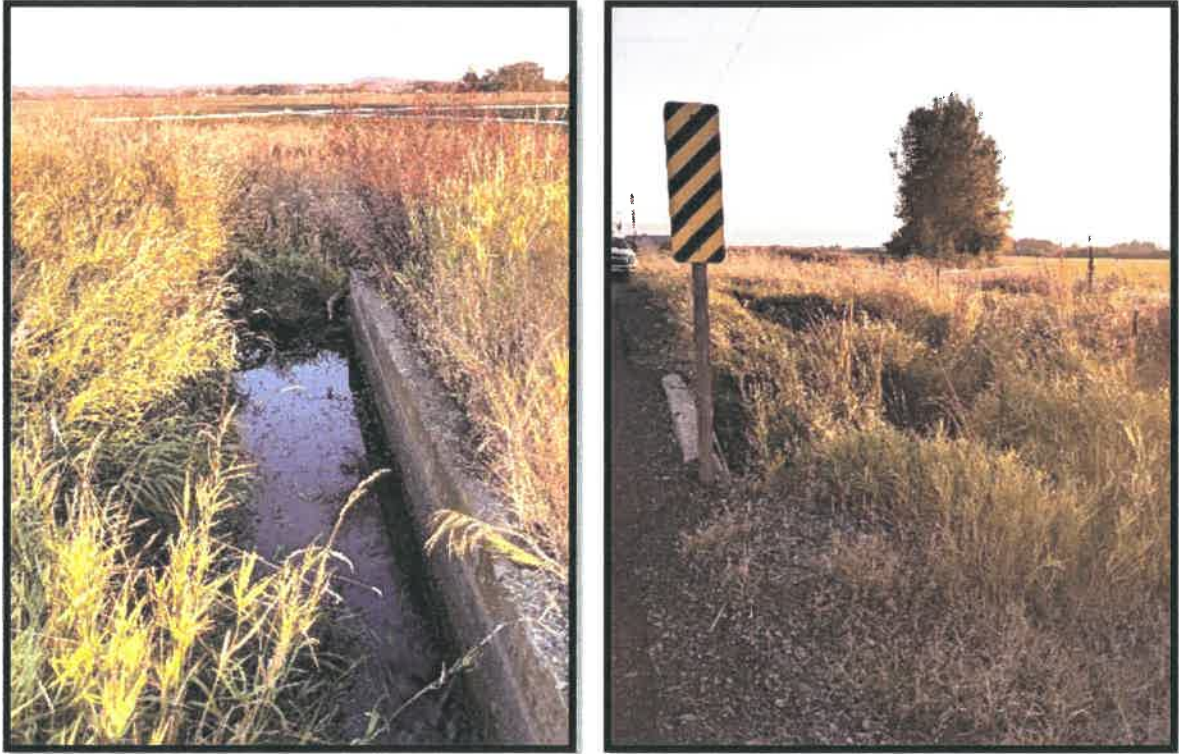
Figure 3. Photos of Coleman Creek Segment 4 looking west from Fairview Road at outlet from Culvert 3 (left) and south at Coleman Creek as it exits the project limits (right).
